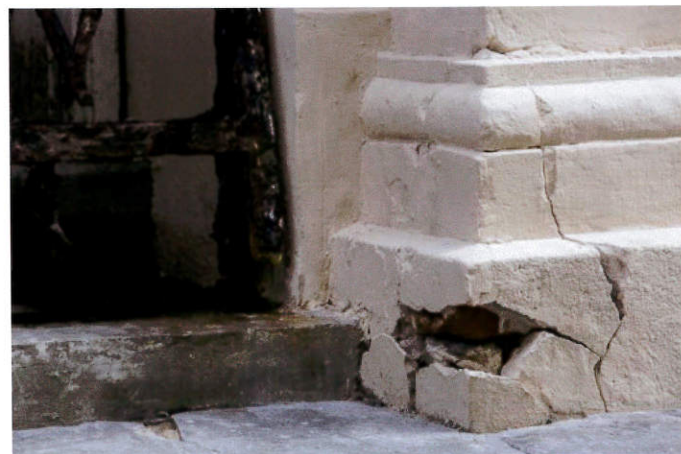
E3A1998 - Exterior: detail of side entrance gate area along Pere Antoine Alley
